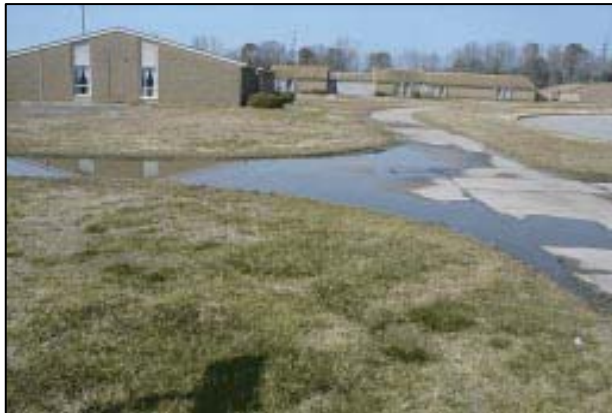
Excessive ponding of water on sidewalks. Poor drainage makes walkways impassible for residents.
