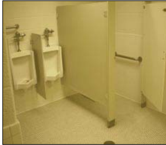
Non-ADA compliant restrooms
