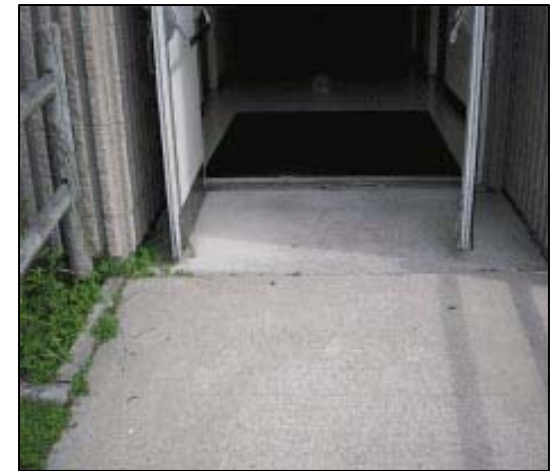
Non-ADA compliant entrances/exits
