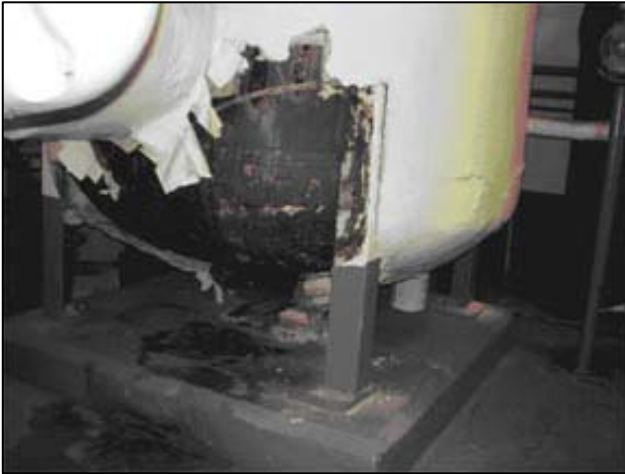
Hot water tank rusting through at drain plug, beyond useful life.
