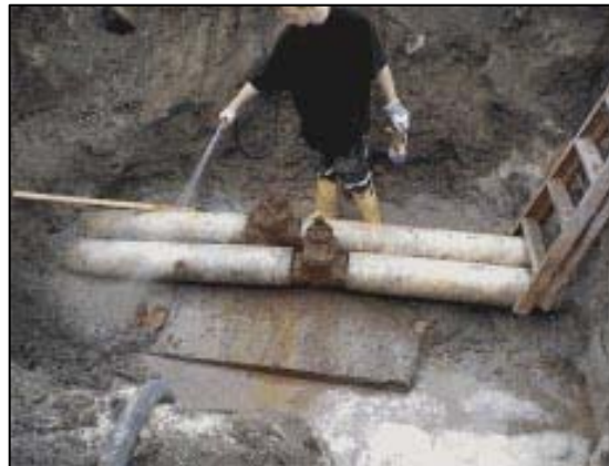
Stress crack on 8 inch water main required shutdown of entire facility due to faulty isolation valves in the ground.
