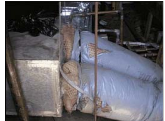
HVAC & duct work at end of useful life
